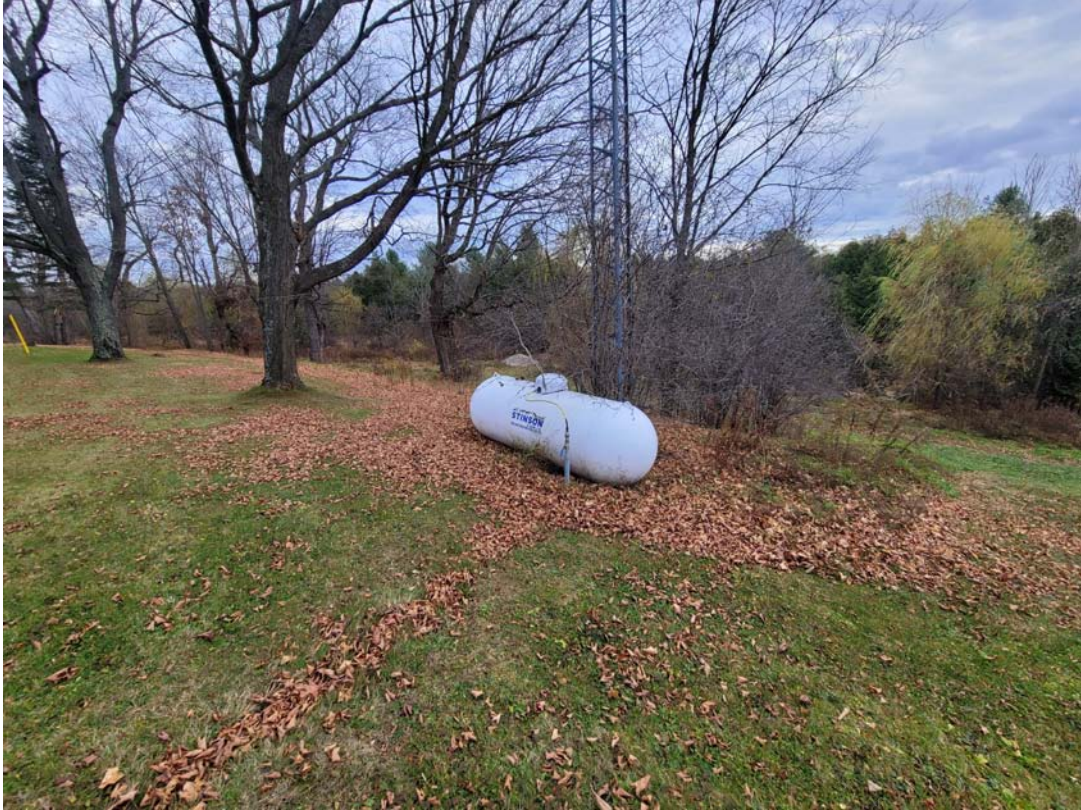
View of above ground propose storage tank
