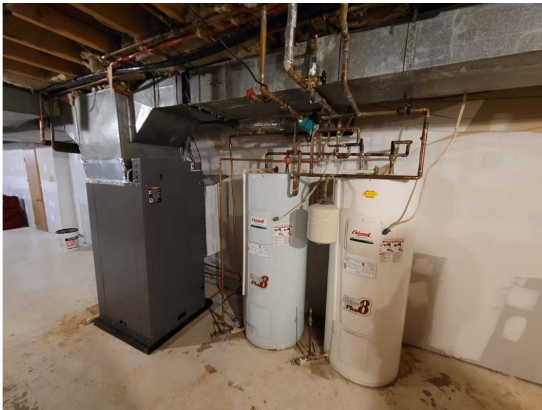
View of geothermal heat pump in basement of single family dwelling
